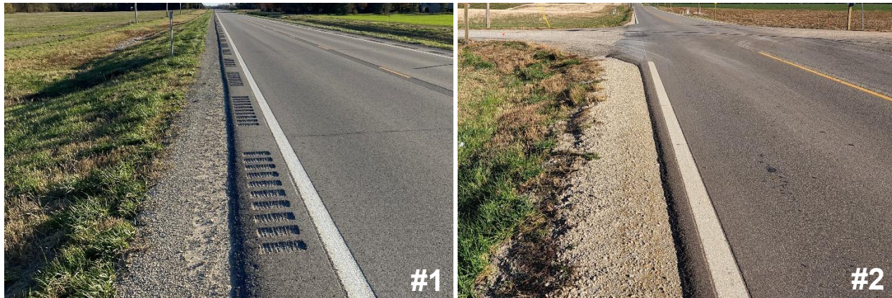
Figure 3 – Shoulder Condition Photos
